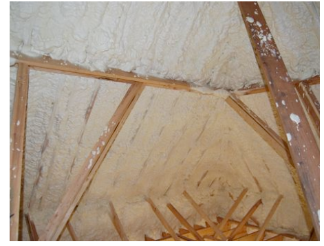
Roof deck is sprayed at 5.5"+ creating an unvented and "close to room temperature" attic.
