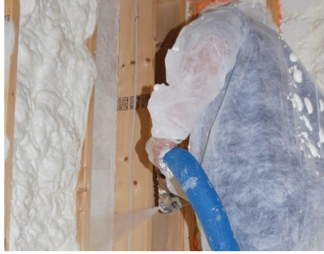
3.5" of Icynene out performs R19 of fiberglass or wet cellulose in walls.
